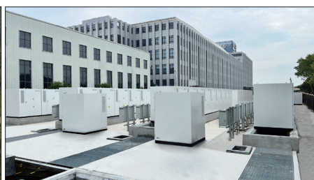
Commercial and Industrial Renewable Energy with Storage
